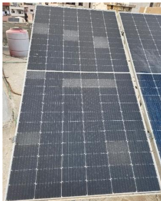
Figure 4: The studied PV solar system at the second measurement number2
