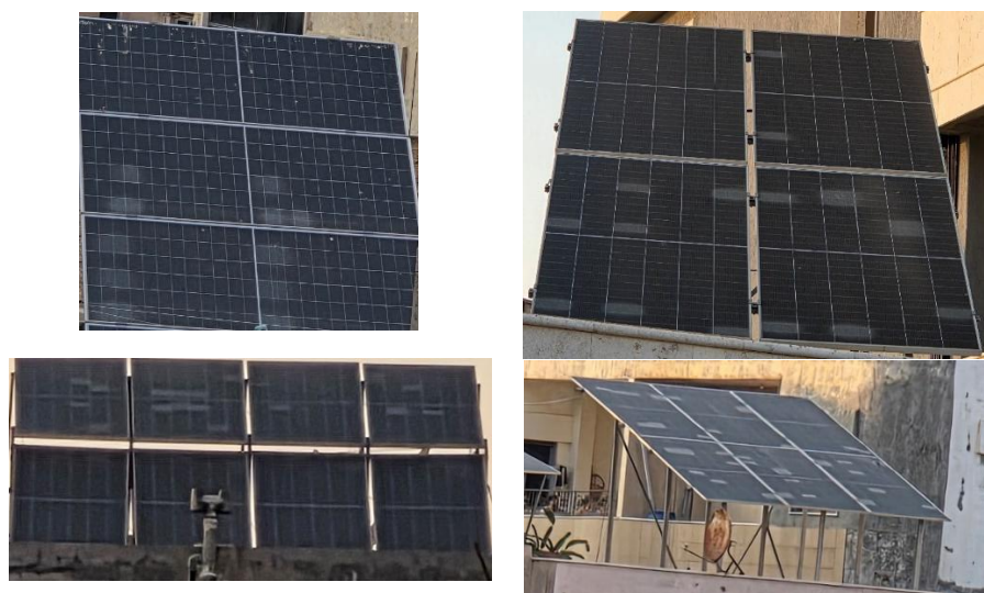
Figure 3: The phenomenon on other nearby rooftop PV systems
