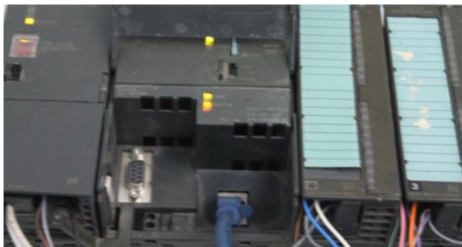
Figure 15. PLC Ethernet module light indicator status.
