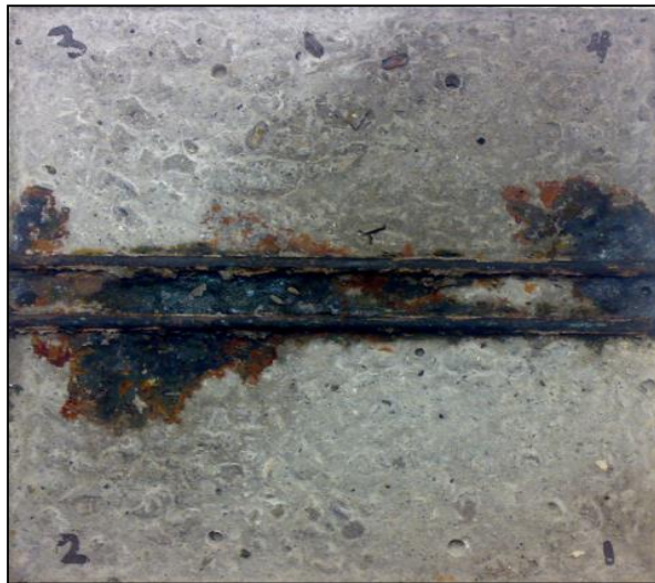
Fig. 12: Photo of the upper concrete surface and corroded wires
